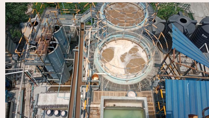
Effluent Treatment Plant at Pantnagar Unit
