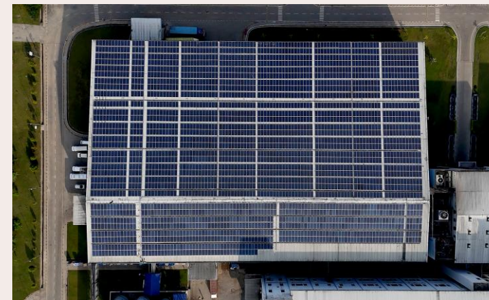
Solar Panels installed at Pacharia Unit
