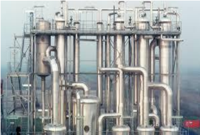
Zero Liquid Discharge Plant
