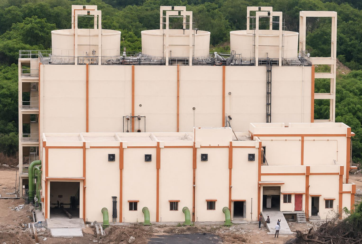
Cooling Tower with Water Recirculation Plant, RINL Capacity : 7500 m3 / hr
