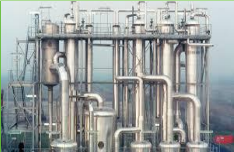
Zero Liquid Discharge Plant
