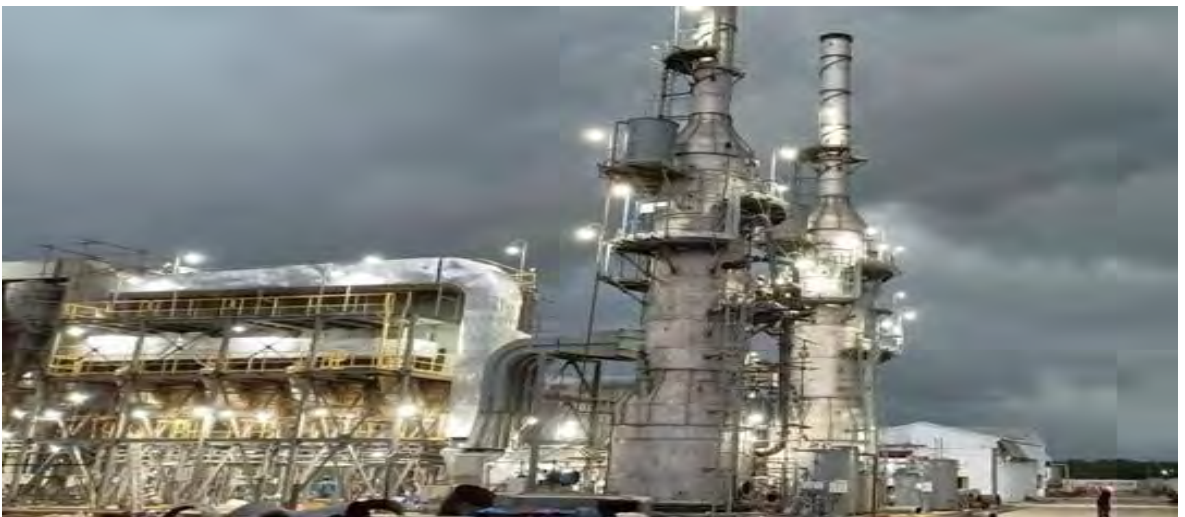
(India's first FGD in Battery Breaking unit at Haldia, West Bengal.)
