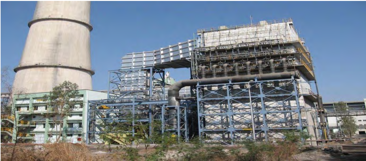
(India's first sea water FGD system with 100% of flue gas for 2 x 250 MW Dahanu Thermal Power Station at Dahanu, Maharashtra, India, installed by our Company.)
