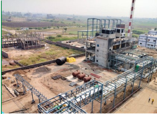
Utility, Common Tank Farm & IB Yard
