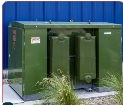
Pad Mounted Transformers
