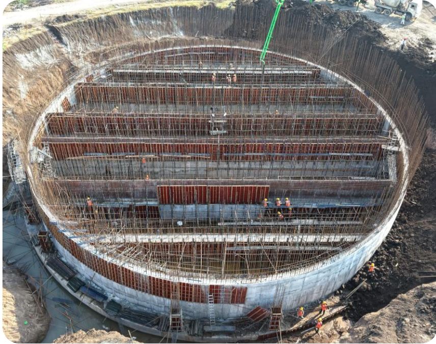
Clinker Silo Pune Grinding Unit (Expected commissioning: Q2 FY28)
