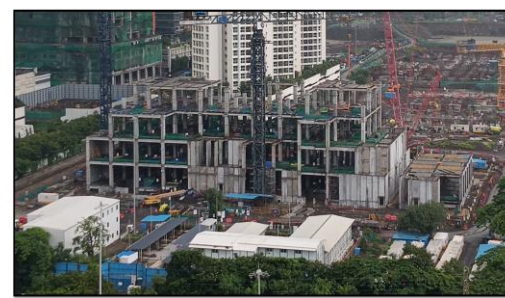
Data Center, Maharashtra
