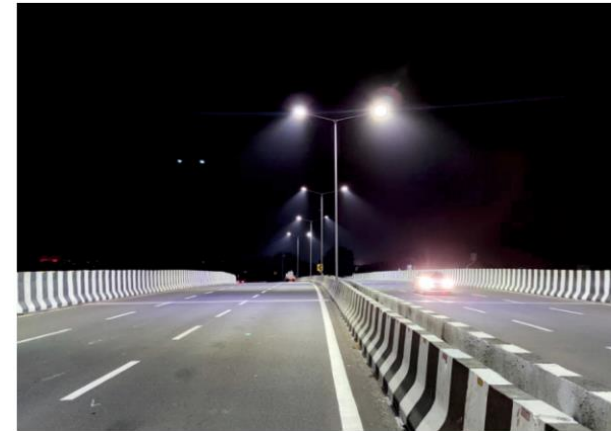
Complete Highway Lighting System, NH-16
