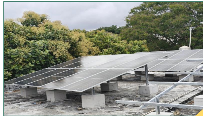
Ongoing Rooftop Solar installations for Indian Railways, South Western Railway - Mysore Division
