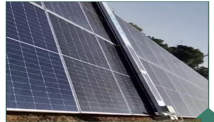
Use of robotic cleaners on the 944 KWp DC solar plant to maximize power generation efficiency.
