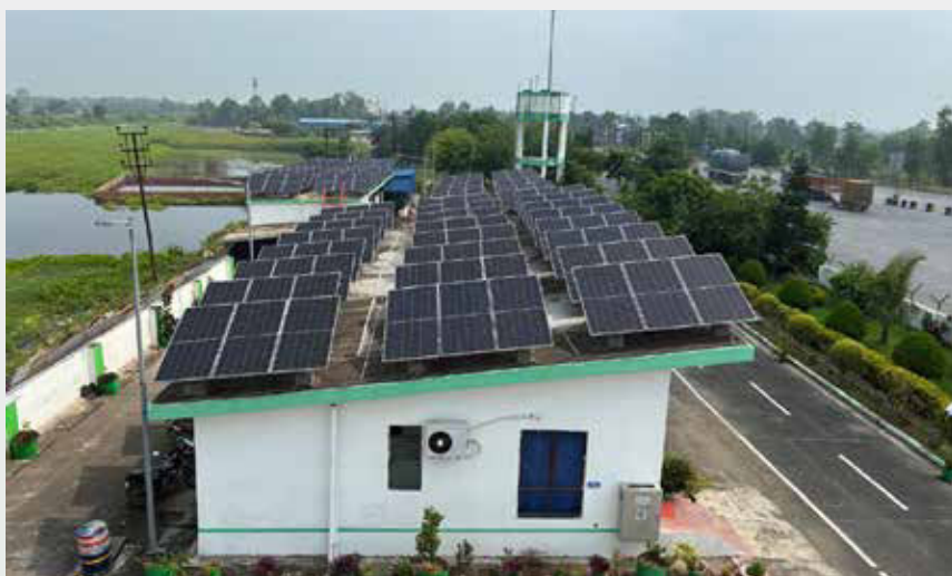
Installed Solar Panel at FRHPL
