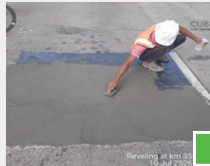
Treatment for Raveling in Rigid Pavement
