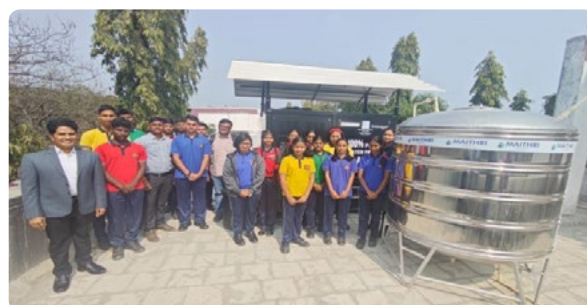
Atmospheric Water Generators (AWG) system at Kendriya Vidyalaya, Dundigal, Hyderabad.
