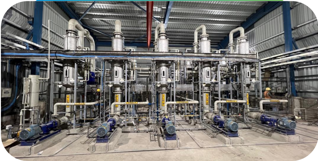
Waste Heat Evaporators
