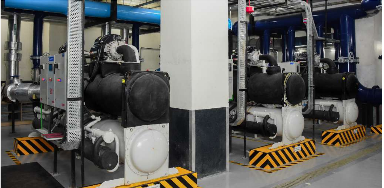
Magnetic bearing oil-free chillers and MEP works at Meenakshi Super Specialty Hospital, Madurai
