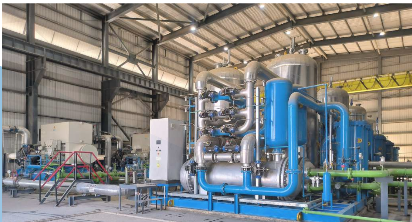
Compressed air station at Kutch Copper Limited, Gujarat
