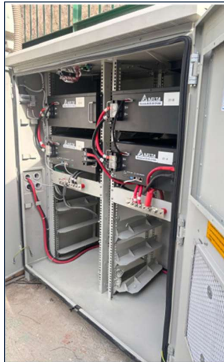
314 AH Lithium Battery- POC
