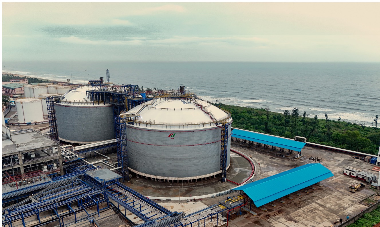
Operational LPG terminal at New Mangalore Port Authority
