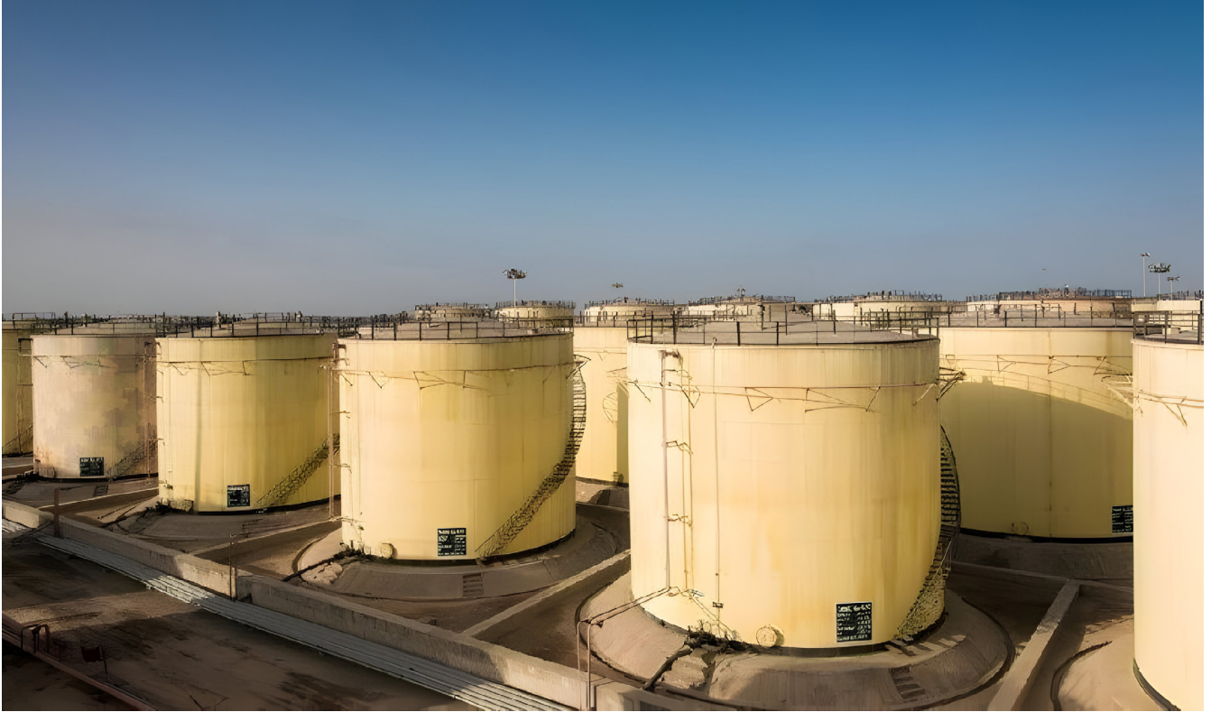
Liquid tank unit at Kandla Terminal-4
