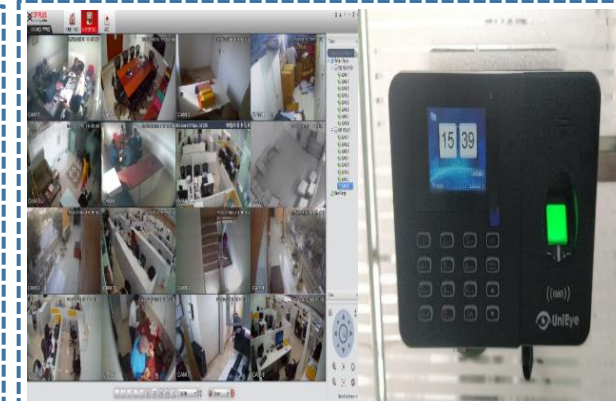
Fully CCTV enabled warehouses & branch network with biometric machines
