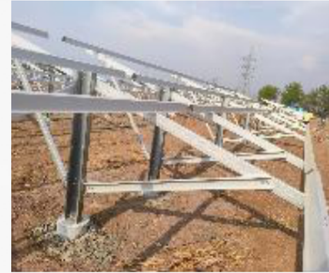
Solar frame structure
