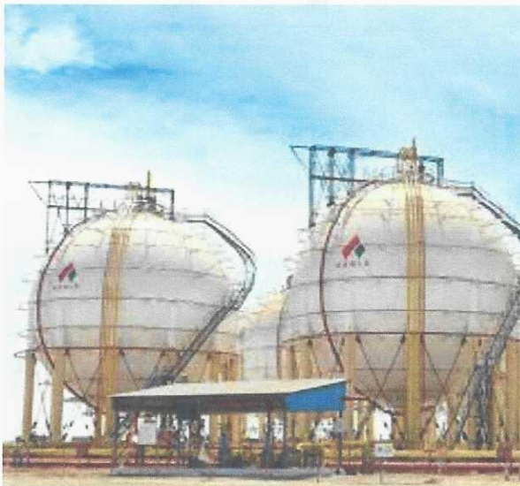
SPHERICAL TANK FOR LPG STORAGE
