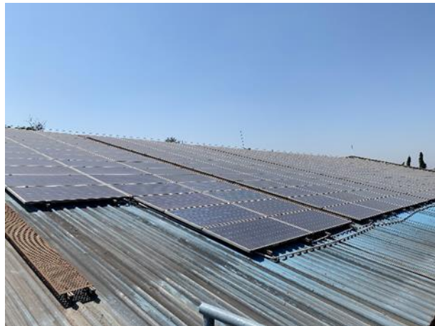
SOLAR POWER PANELS
