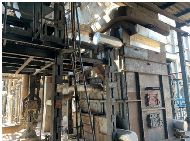
2 X 10 TPH Boilers
