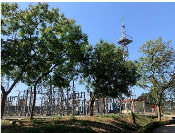
66 KV SWITCH YARD
