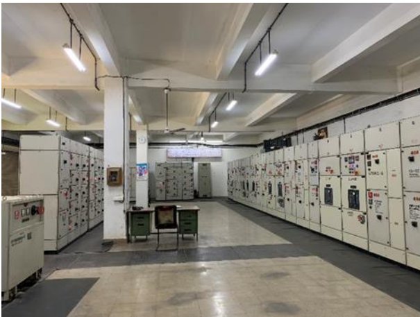
MAIN POWER PANELS
