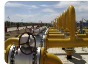
City Gas Distribution
