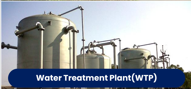
Pre-treatment Clarification & Pumping System
