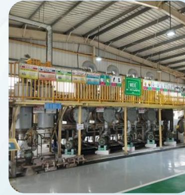
Zero Liquid Discharge Plant
