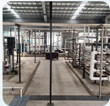
Multiple Reverse Osmosis Plant
