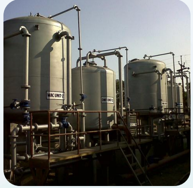
Water Treatment Plant (WTP)
