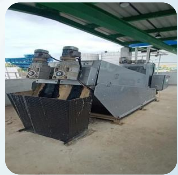
Sludge Dewatering System
