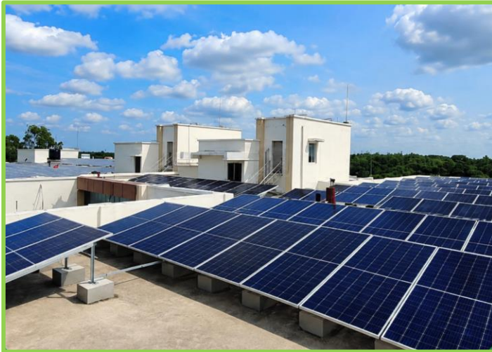
NTPC-SVNIRTAR at Olatpur)
