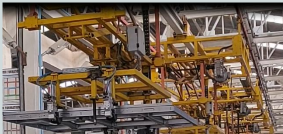
Material Handling System for Line Mode
