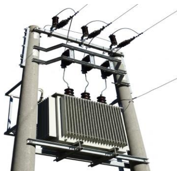
EPC RDSS (Revamp Distribution Sector Scheme)
