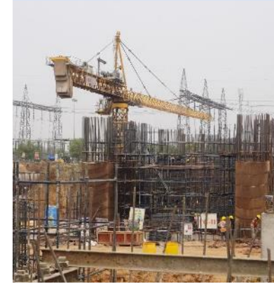
Unit #3 - Turbine Generator Deck
