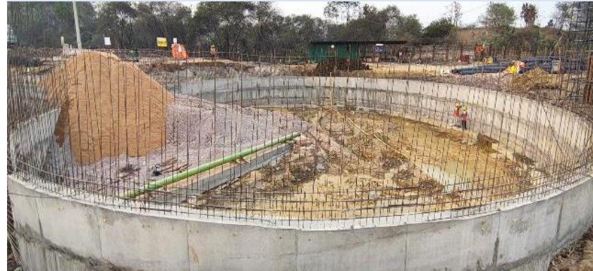
High-Rate Solid Contact Clarifier
