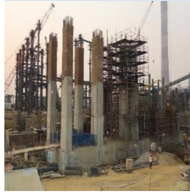
Unit #3 - Turbine Generator Deck
