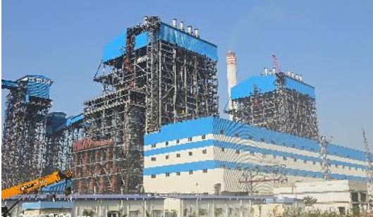
Unit #3 & 4 Boiler Front View
