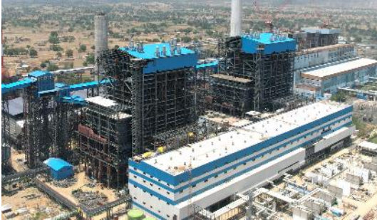
Unit #3 Turbine Bay Overview
