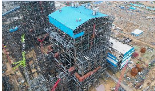
Front View of MPH & Boiler
