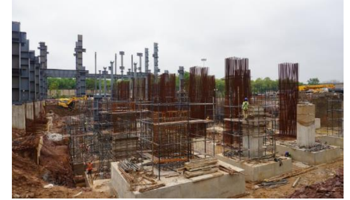
Unit #3 - Turbine Generator Deck
