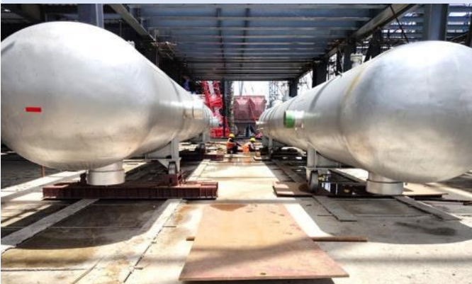
Unit #4 High Pressure Heater
