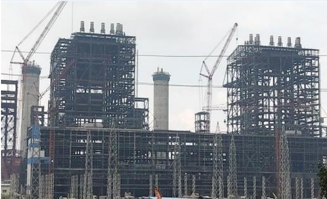
BTG Area Front View
