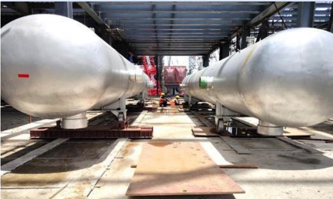
Unit #4 High Pressure Heater
