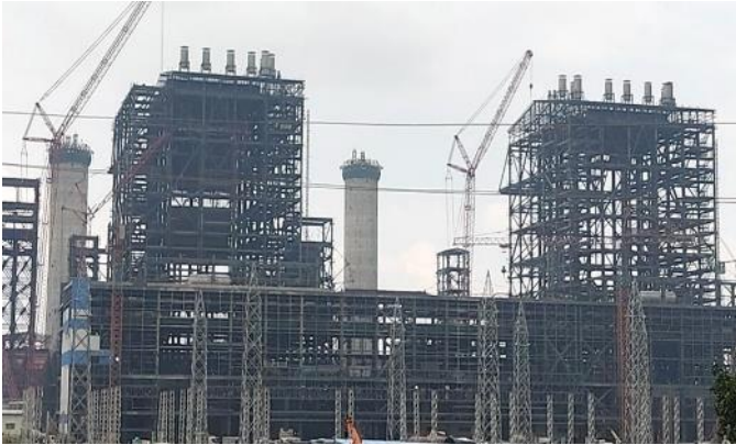
BTG Area Front View
