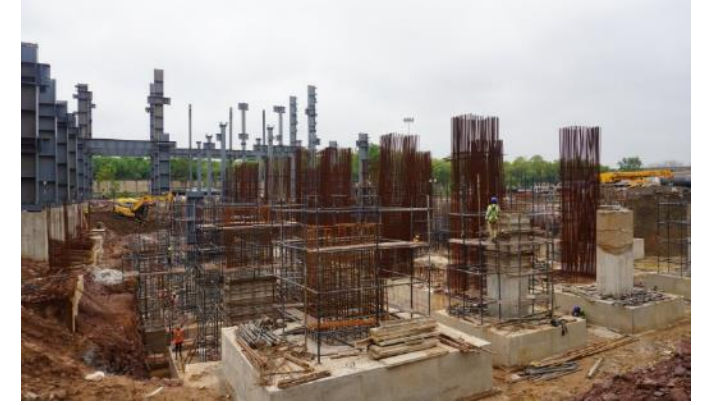
Unit #3 - Turbine Generator Deck
