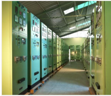
Control Relay Panels
