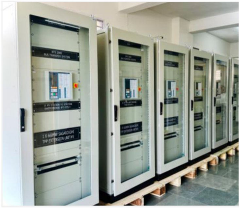
Bus Transfer System
