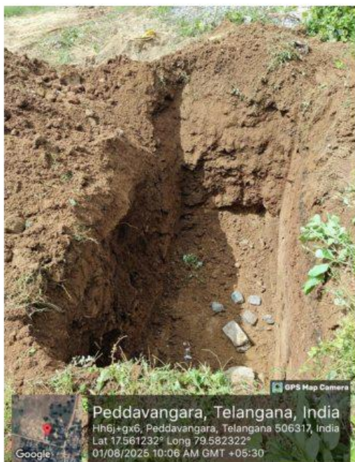
ZPHS PEDDAVANGARA SCHOOL RAINWATER HARVESTING 01.08.2025.
