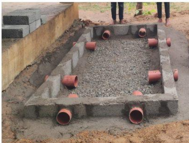
Rain Water Harvesting pit
