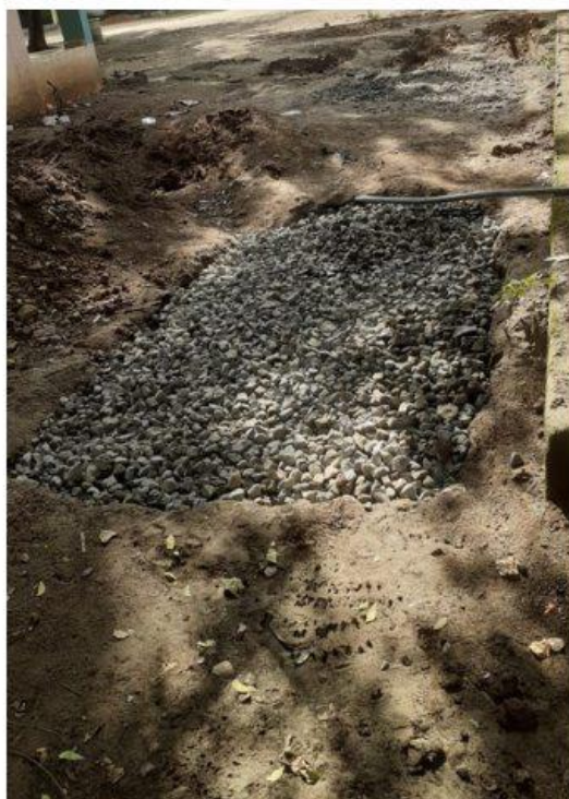
Rain Water Harvesting pit
