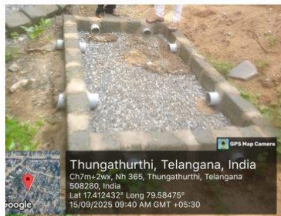
Rain Water Harvesting pit on 15.09.2025
