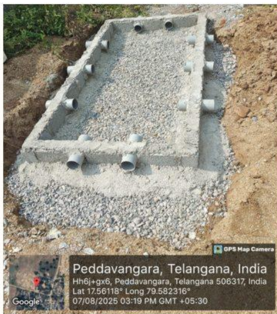
Rain water Harvesting Pit 07.08.2025
