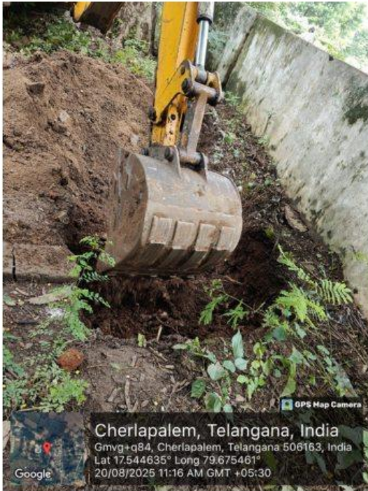
ZPHS Cherapalem School Rainwater harvesting pit 20.08.2025
