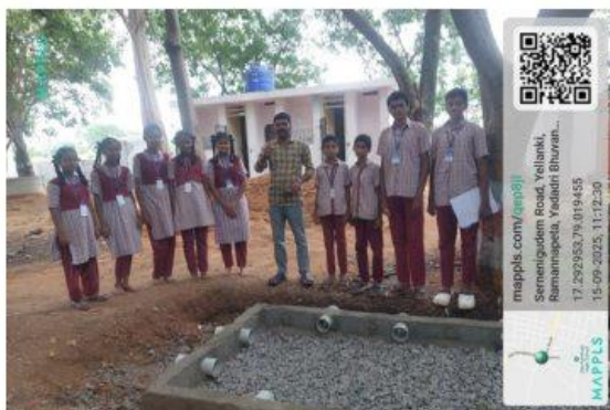
Rain Water Harvesting pit 15.09.2025
