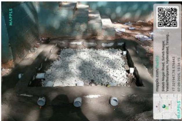
Rainwater Harvesting Pit at ZPHS Sahebnagar School, Rangareddy District. 07.09.2025
