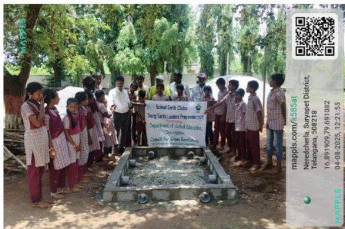
Rain water Harvesting Pit 04.08.2025.
