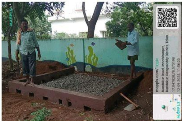
Rainwater Harvesting Pit 12.09.2025
