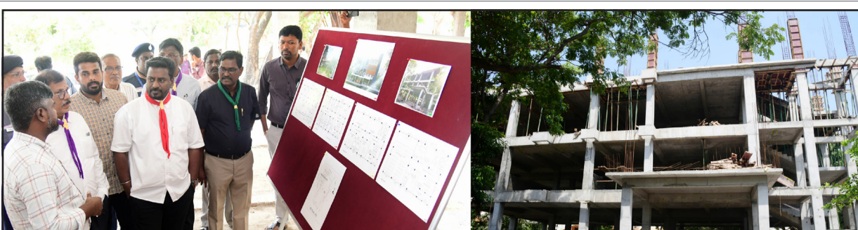
School Education, Tamil Development, Information and Publicity Minister Raj Mohan inspected the construction works of the new Bharat Scouts and Guides State Headquarters building being constructed at a cost of Rs.8.93 crore in Kamarajar Salai, Chennai. School Education Director S. Kannappan, Elementary Education Director P.A. Naresh, Assistant Executive Engineer Senthil Raj, Assistant Engineer Tamilarasi, and senior government officials accompanied him during the inspection.
