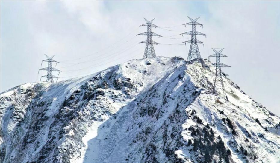
400 kV Samba Amargarh
