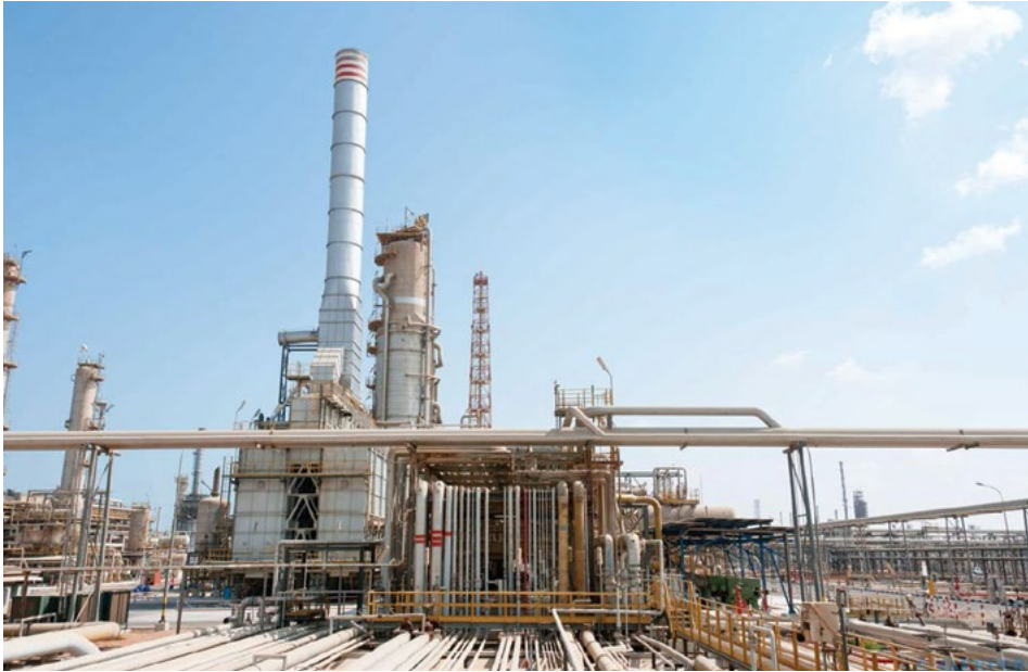
Ruwais and Abu Dhabi Oil Refinery
