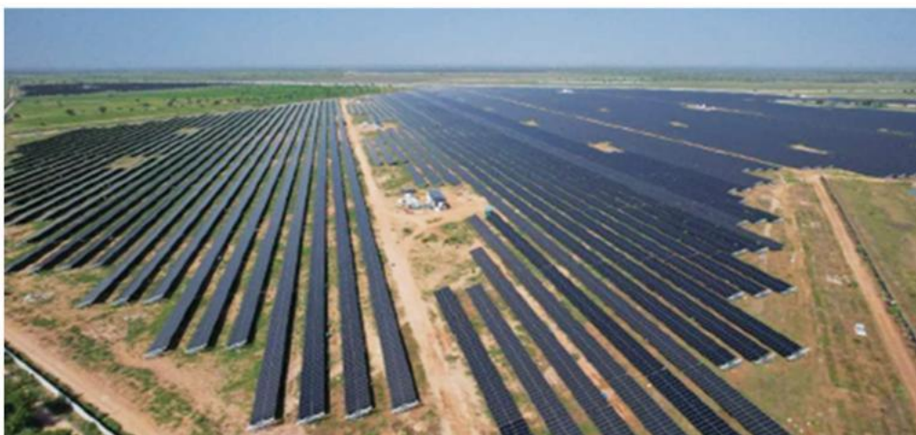
300 MW Solar Power Project located in Phalodi District, Rajasthan
