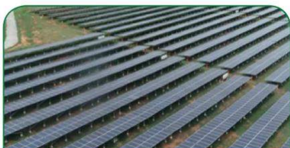
10 MW Solar PV Power Plant at Defence Research and Development Organisation (DRDO) premises, Kolar, Karnataka
