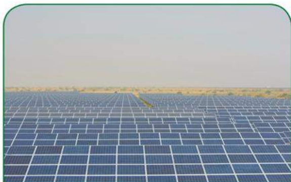
10 MW Solar PV Power Plant at Badi Sid, Rajasthan
