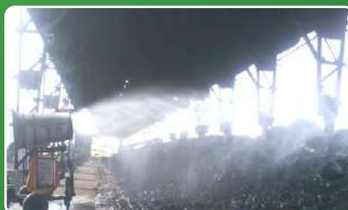
Mobile dust suppression system in track hopper area in CHP to control fugitive dust
