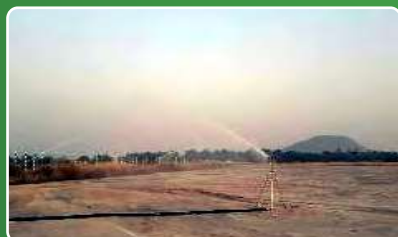
Ash pond dust suppression system around ash pond to control fugitive emission
