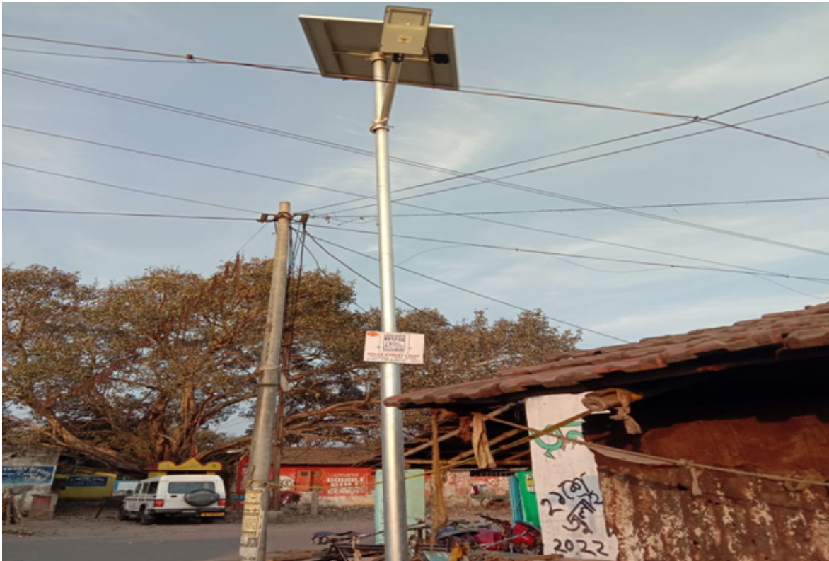
Solar Street light installed at Village Sukantopally: CSR, Durgapur TPS
