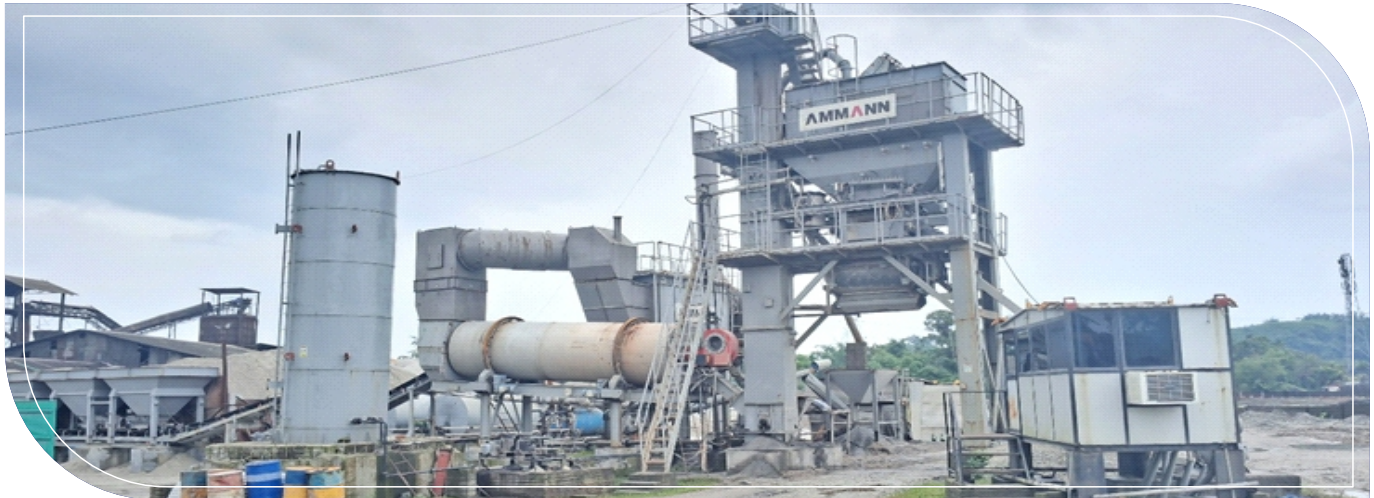
WET MIX MACADAM PLANT
