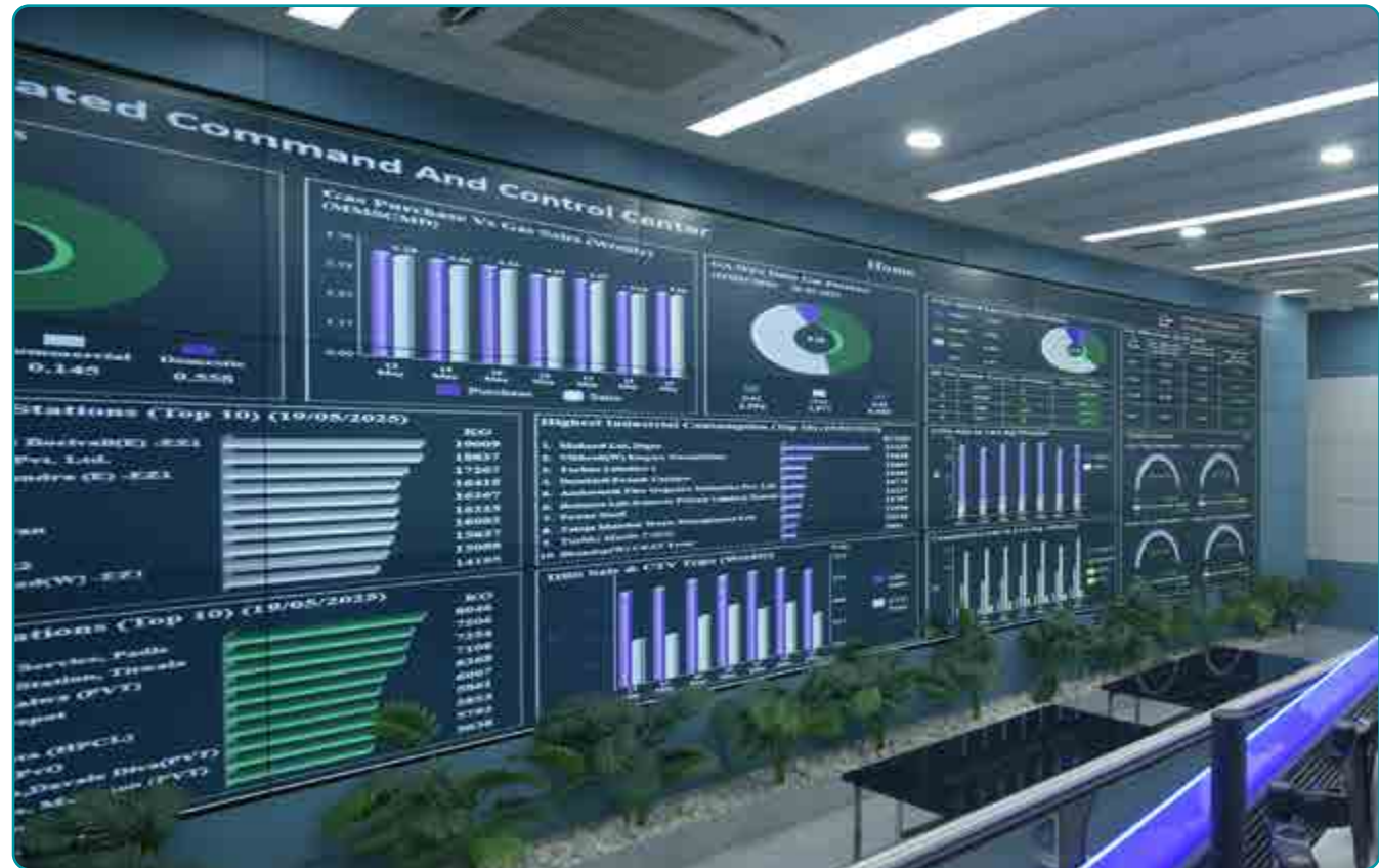
➤ The Integrated Command and Control Centre at MGL Mahape Office
