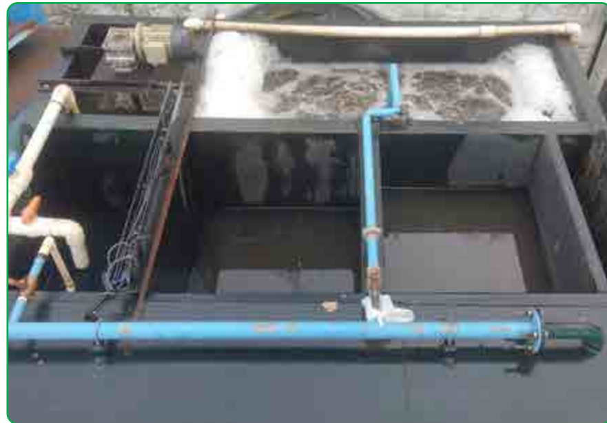
➤ Sewage Treatment Plant installed at CGS Mahape
