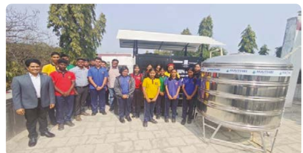
Atmospheric Water Generators (AWG) system at Kendriya Vidyalaya, Dundigal, Hyderabad.
