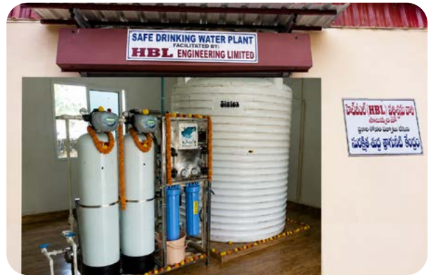
Community level Safe Drinking Water Plant Setup in Vizianagaram District, Andhra Pradesh
