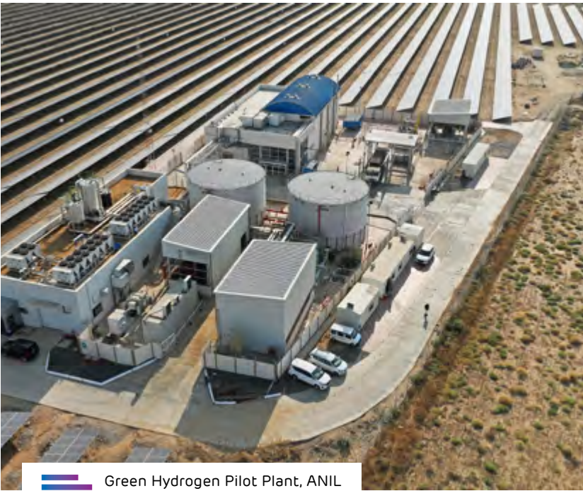
Green Hydrogen Pilot Plant, ANIL
