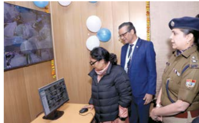
CCTV Surveillance System installed & commissioned by BEL in Kotdwara, Uttarakhand, was handed over to Kotdwara State Police in the presence of Hon'ble Speaker, Uttarakhand Legislative Assembly
