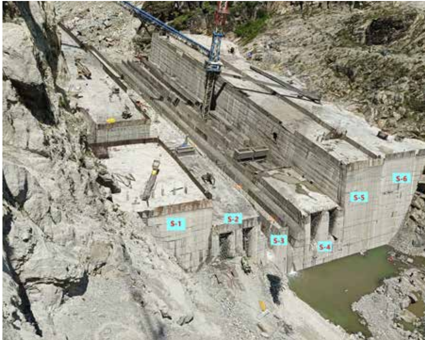
CONCRETING OF 135 M HIGH CONCRETE GRAVITY DAM – 624 MW KIRU (UT OF J&K)
