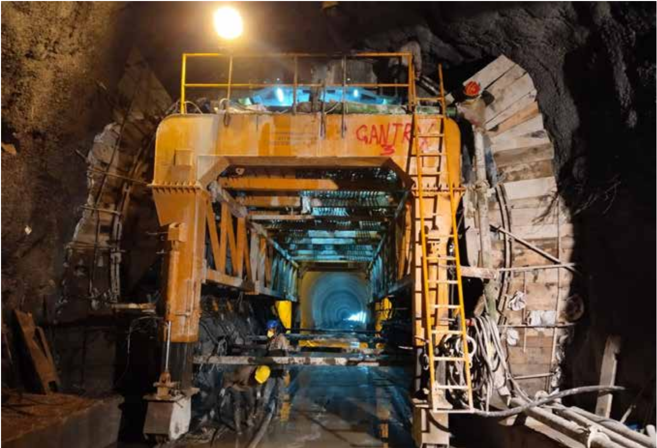
LINING WORKS IN FACE-3 & FACE-4 OF HEAD RACE TUNNEL – 800 MW PARBATI-II (HIMACHAL PRADESH)
