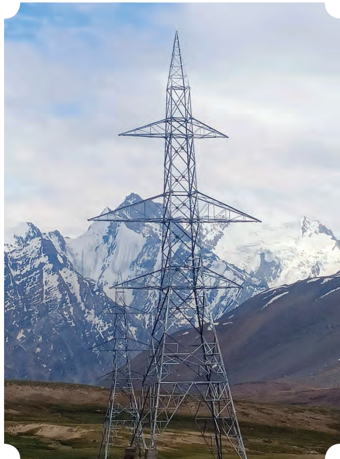
220kv Single Circuit Transmission Line from Drass to Padum on Double Circuit Tower at Kargil, Ladakh being implemented by RECPDCL
