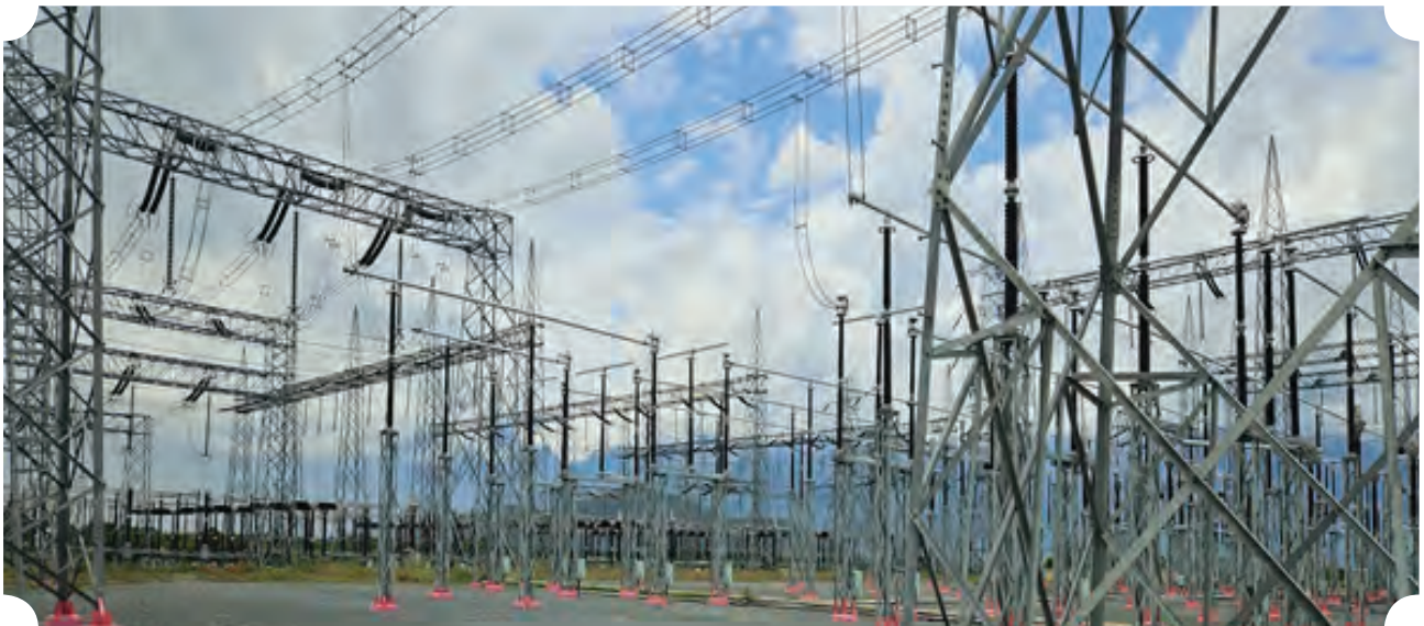
Karamadai 400kV Substation Bay extension of Kundah Power Evacuation project (Tamil Nadu) financed by REC
