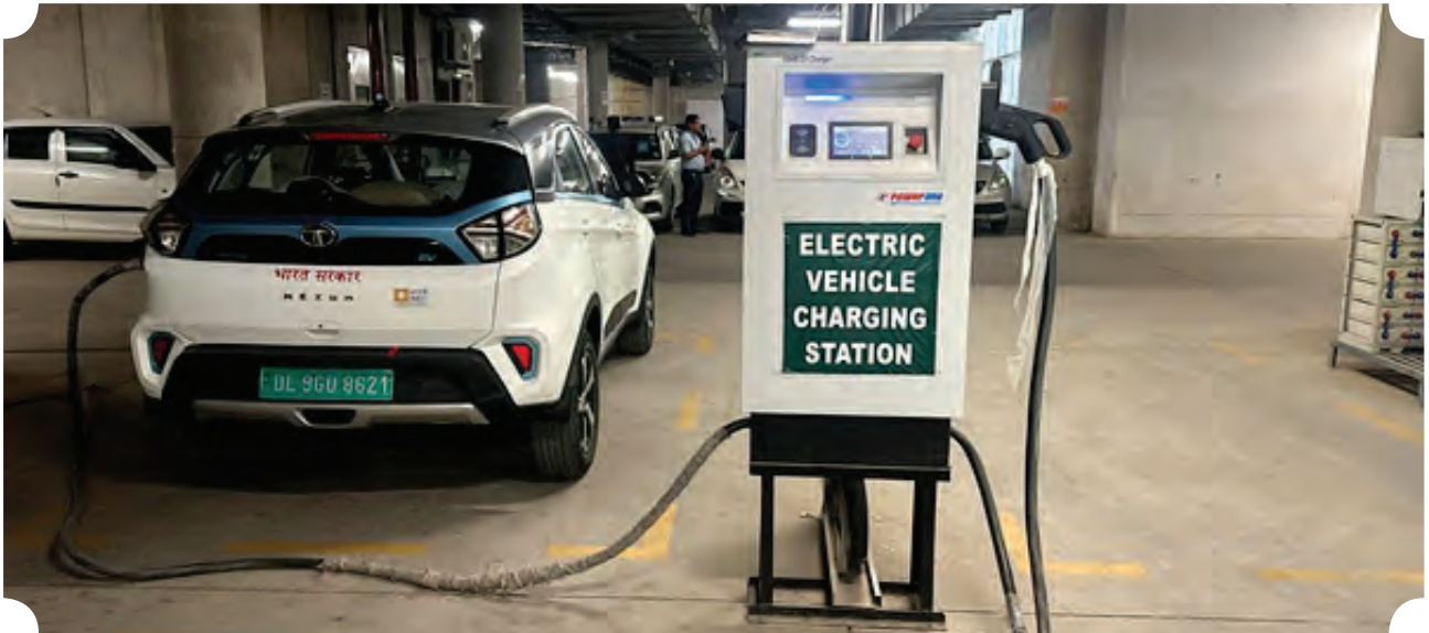
EV charging station at REC Corporate Office, Gurugram
