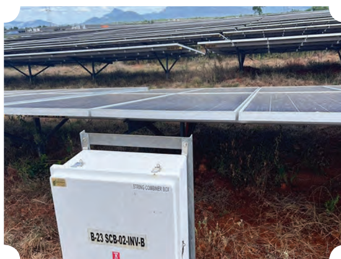
100 MW (110 MWp) Solar PV Project in Theni / Batlagundu, Tamil Nadu financed by REC
