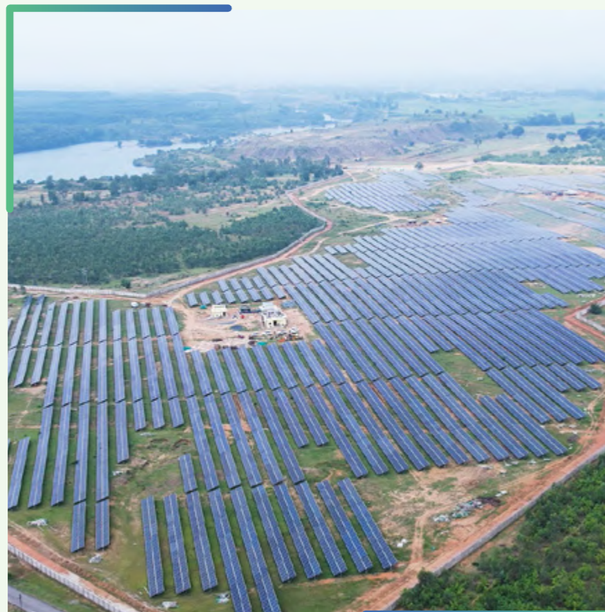
● 20 MW Ground Mounted Grid connected Solar Power Plant
