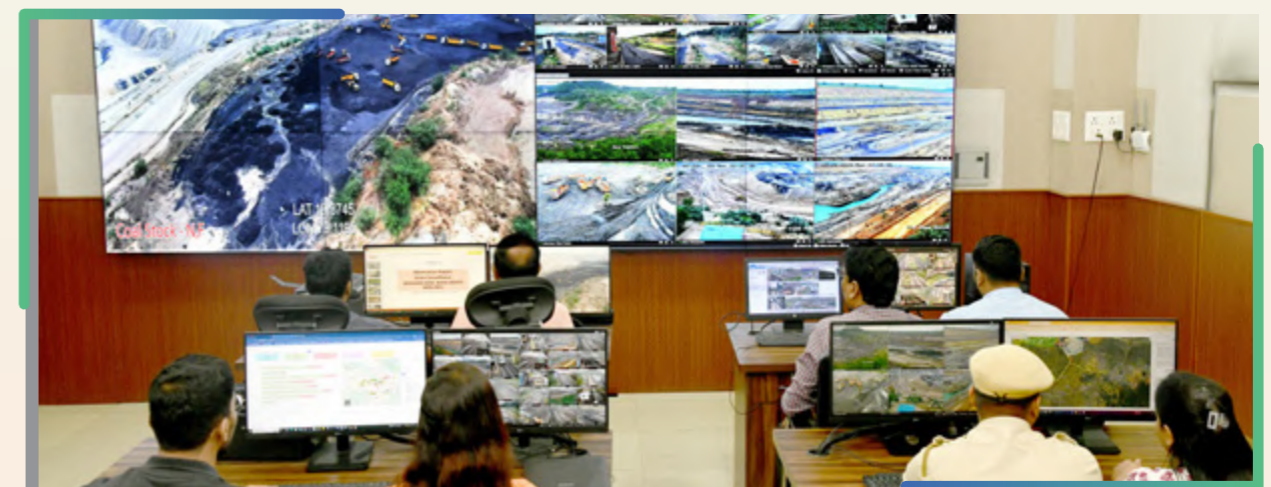
● Integrated Command and Control Centre at WCL Headquarter
