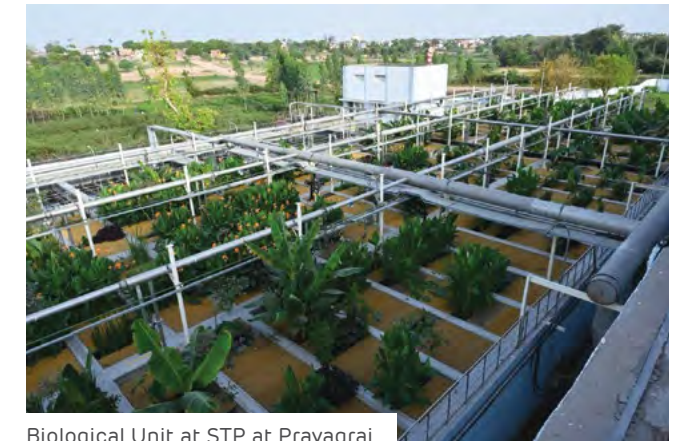
Biological Unit at STP at Prayagraj
