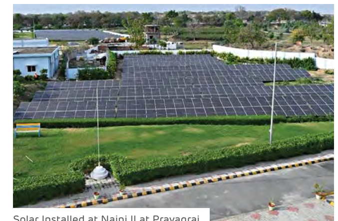
Solar Installed at Naini II at Prayagraj
